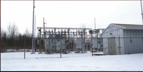
Substations contain high-voltage electricity.
