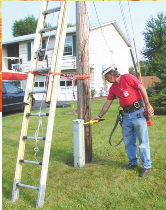
A worker uses a voltage tester to re-test telecom pedestal on joint-use pole.
