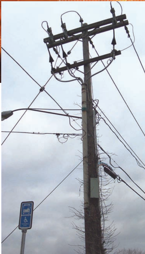
Moisture-laden vines on poles that cross power lines and are in telecom space create electrical risks. The protruding cable box represents another hazard for workers climbing the pole.
