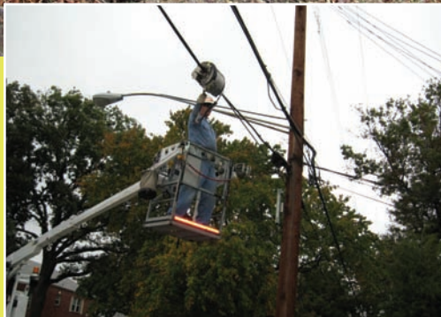
Working near power lines, a technician uses a lasher to join telecom lines.
