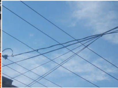
Extreme risk: Power lines and telecom lines should never be connected.
