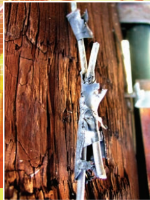
Improper ground on a joint-use pole.
