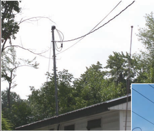
Telecommunications lines should not be attached to an electrical power mast.
